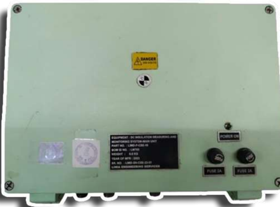
Insulation Monitoring System (IMS)
